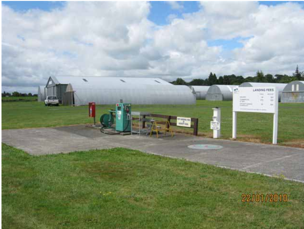
Photo 3: Aviation Fuel pumps and tanks site
